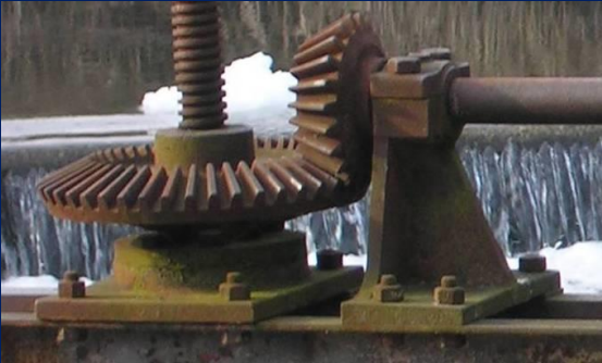
Floodgate power screw operated by bevel gear
